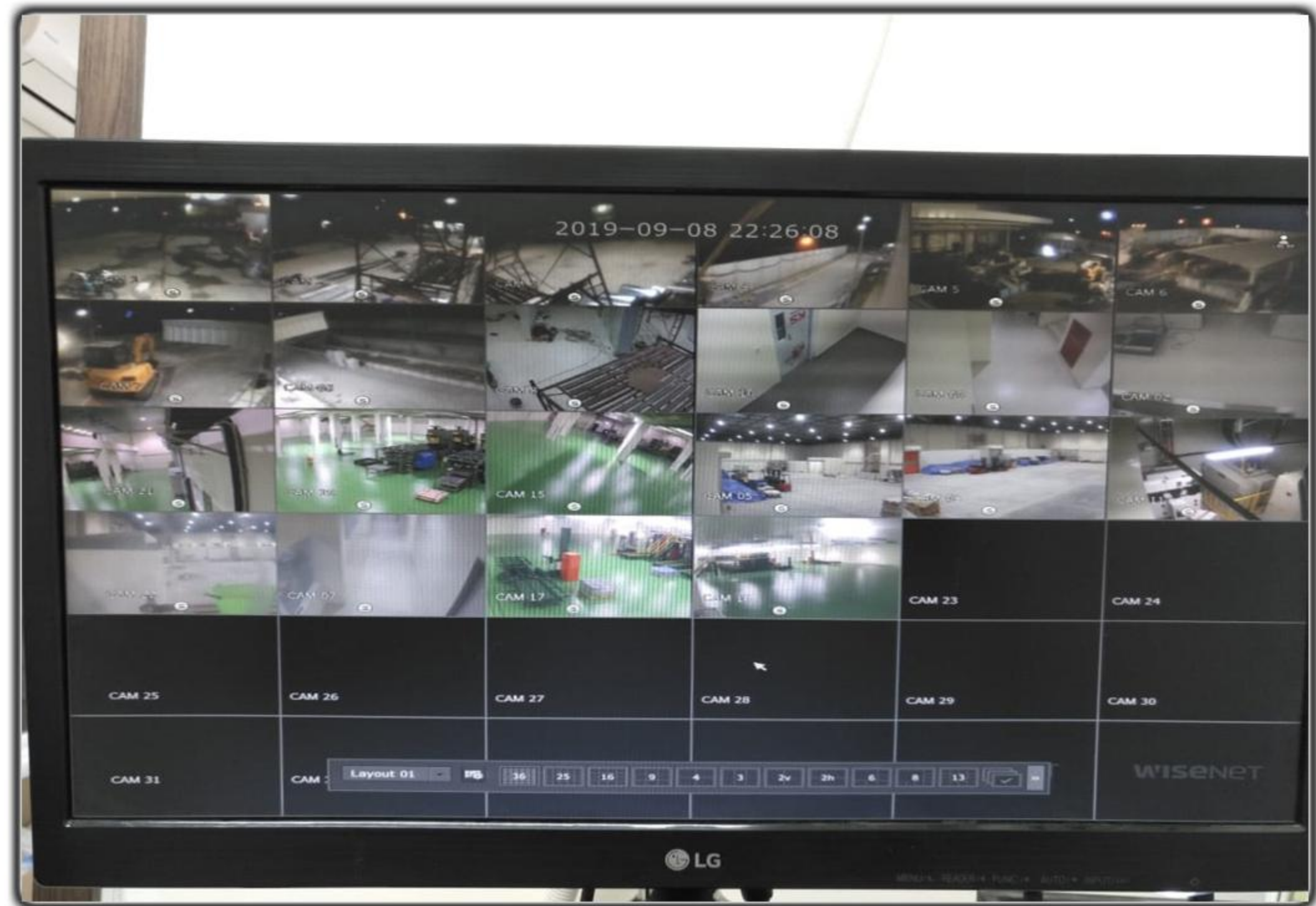
Setting cctv UCC Pandaan
