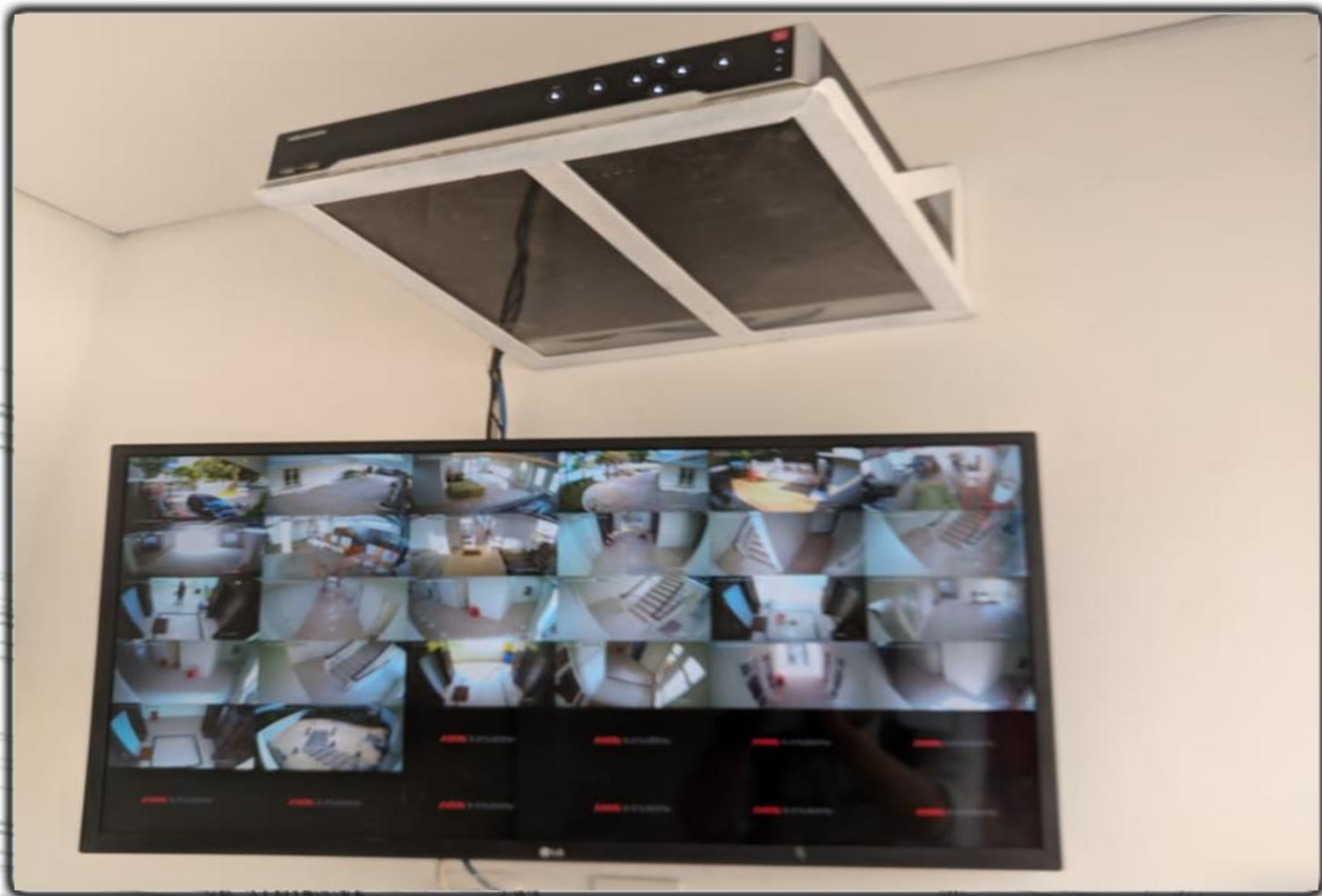
Cctv pos security Thailand Embassy
