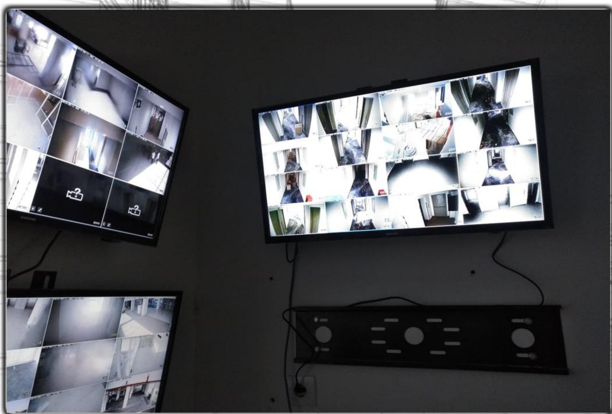
Cctv Hotel Harris
