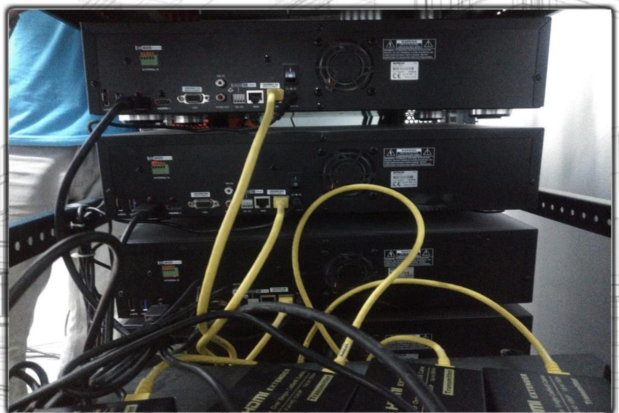
Setting cctv Hotel Harris Surabaya
