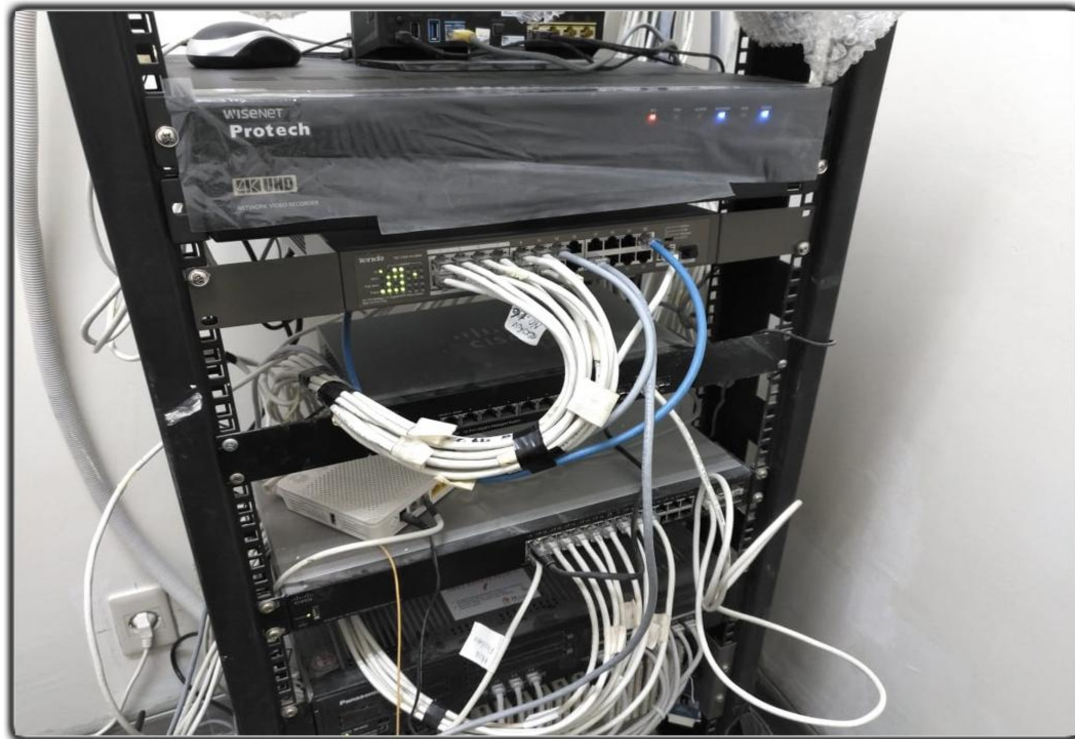
Setting cctv UCC Pandaan
